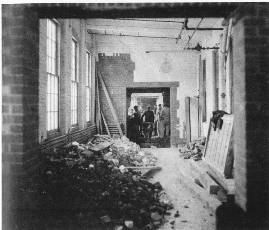
This new passageway for pedestrians, now nearly completed in the ground floor of Building 3, will protect walkers from the heavy truck traffic which fills the roadway between the Blacksmith Shop and Building No. 3.
